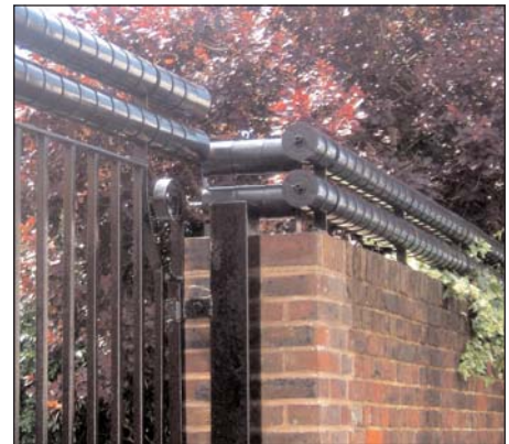
Double row of Roller Barrier, protecting a gate & wall
